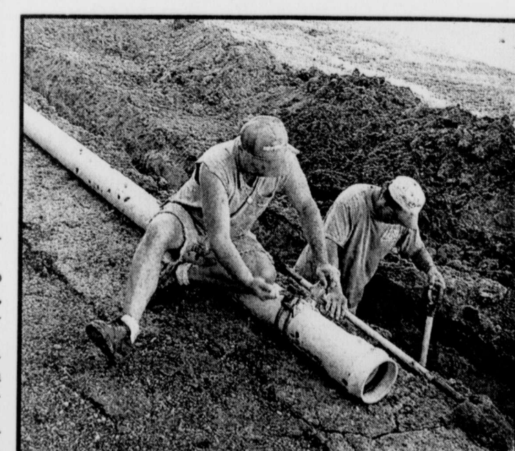
ON LINE Construction Company is nearly finished installing new water lines in the City of Deport. The project is expected to be completed by Thanksgiving. (Staff Photo by Thomas Nichols)
