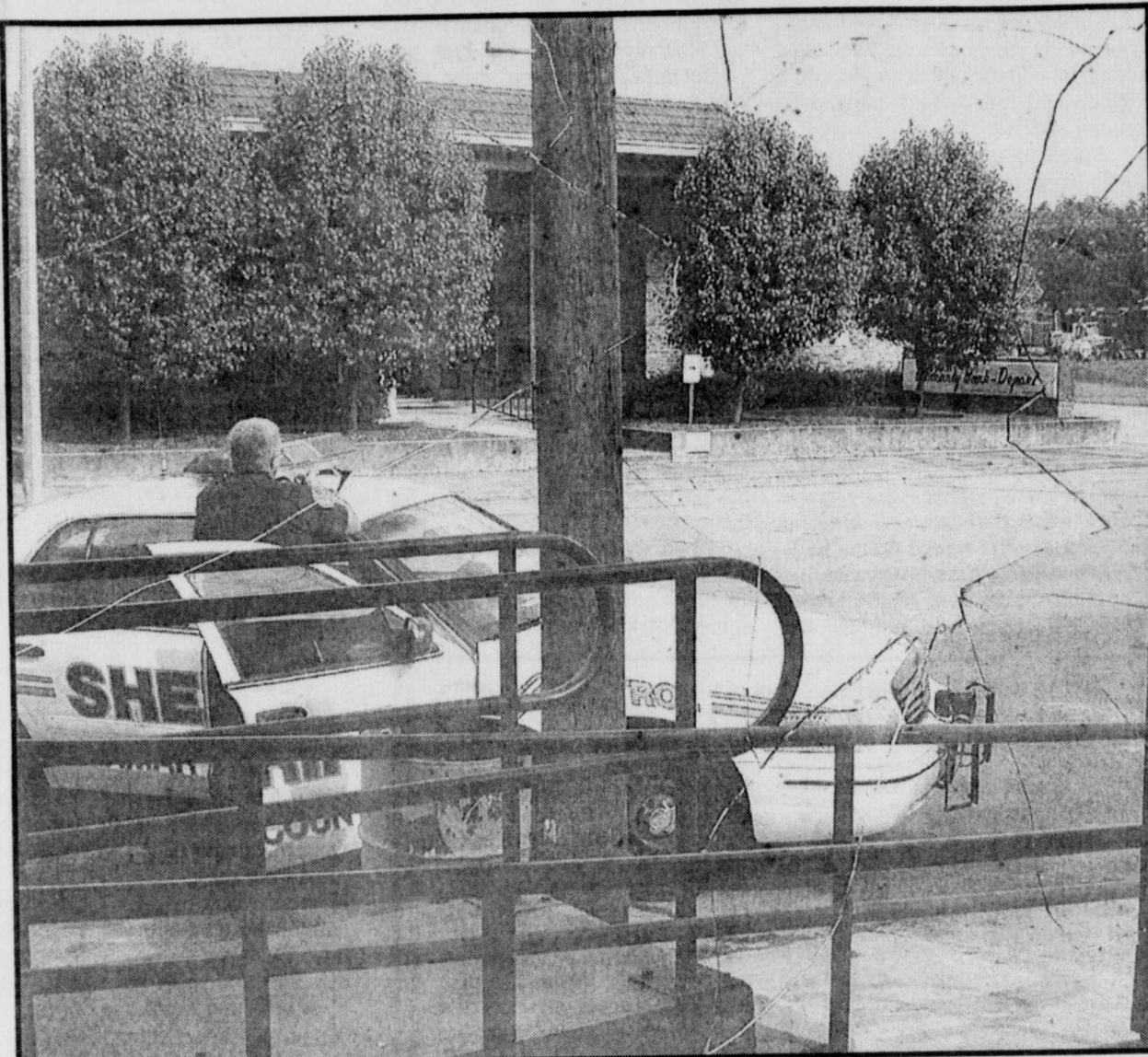
VANDALISM-this window was broken by two juveniles on Sunday, September 1st. The building, which belongs to James and Sunny Whitney, had a large plate glass window broken out. Witnesses identified the two juveniles, who will be doing community service work to make restitution for the window. (Staff Photo by Mike Francis)
