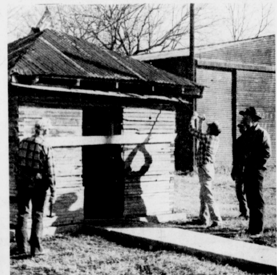
WORKING-The Deport Community Service Club worked on the old jail last Saturday morning they are restoring. They
