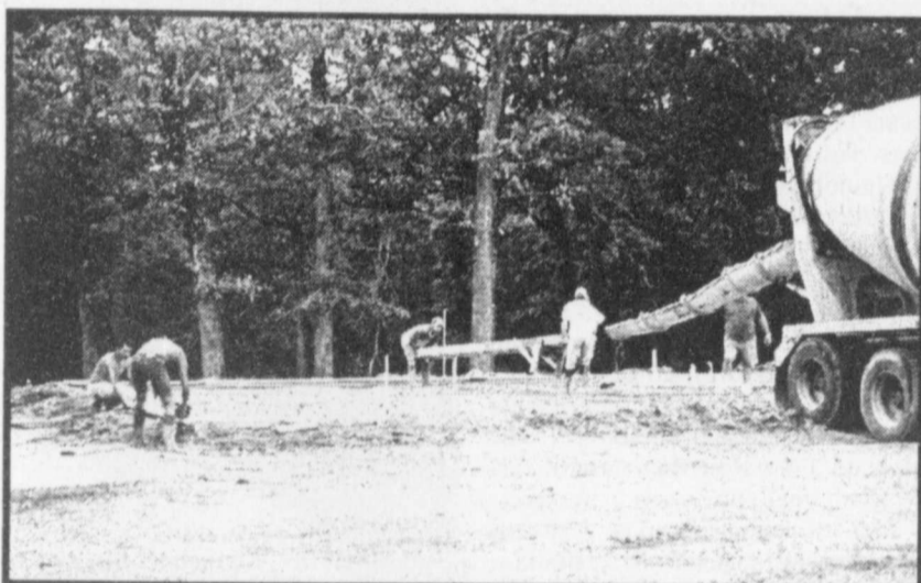
POURING THE FOUNDATION -The foundation was being poured for the new Maple Springs Church Fellowship Hall Tuesday morning. The new building will replace the old church building and will serve not only for the church but for the community. (Staff Photo Nancy Brown)
