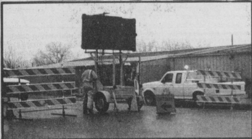
HIGH WATER-forced the closing of Hwy 271 N. of Talco December 27, 2000. Highway Department employees detoured travelers up Fm. 71 west to Hwy. 37 N to Bogata and back onto Hwy. 271 N. (Staff Photo Nancy Brown)
