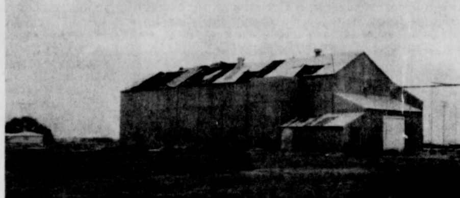
HEAVY RAIN, HIGH WINDS AND HAIL have pounded the Abernathy area since Sunday. In the top photo, taken 3 miles north of town, lake standing from Sunday's storm alone. In the bottom photo, the old gin building just south of Tuco Gin received extensive wind damage Sunday evening. (Review Photos)
