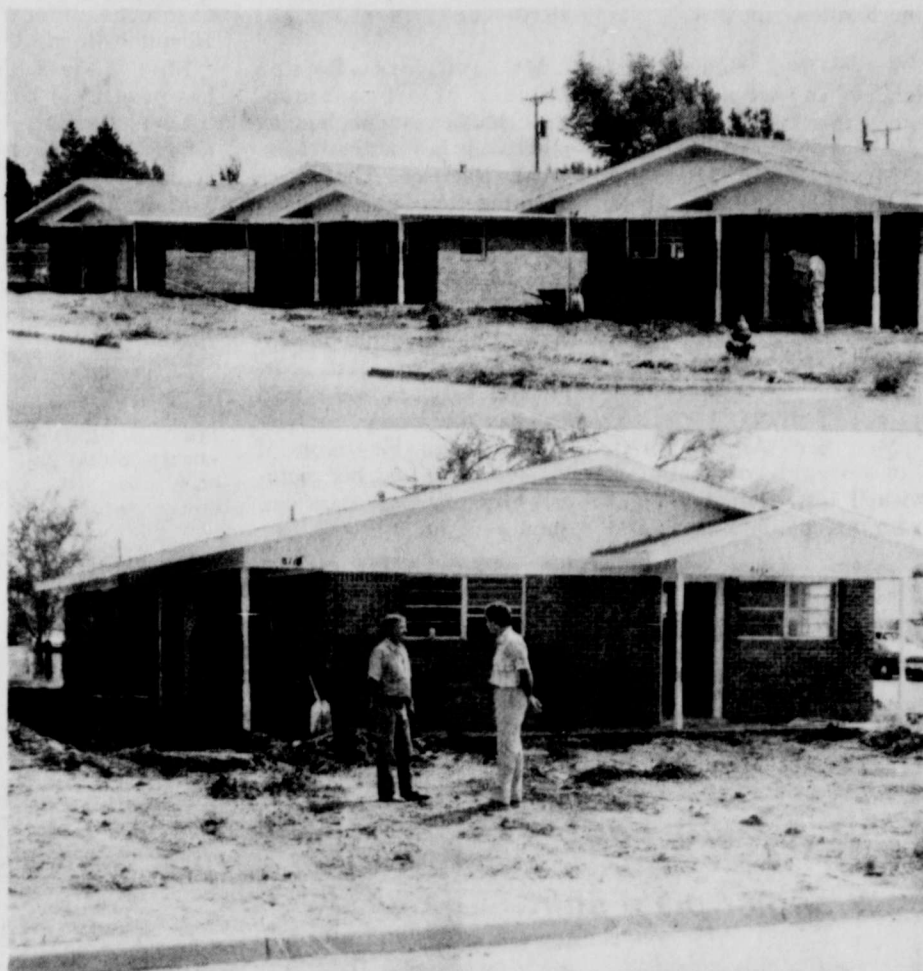
SOON TO BE TOWN HOUSES are the six apartments on the 800 block of 16th Street. They are being remodeled by general contractor Henry Kreiner, pictured in both photos talking to City Manager Rod Ellis. They are pictured standing near the six apartments, which are being converted into town houses. (Review Photos)
