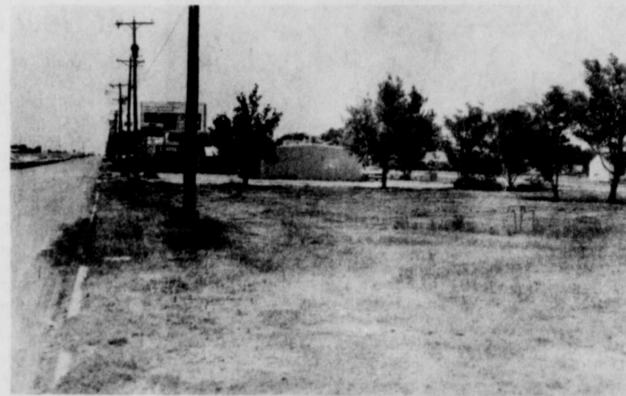
AFTER.... after the substandard house was demolished and removed, a clean mowed lot is the result, thus improving the appearance of Abernathy to viewers from I-27. (Review Photo)
