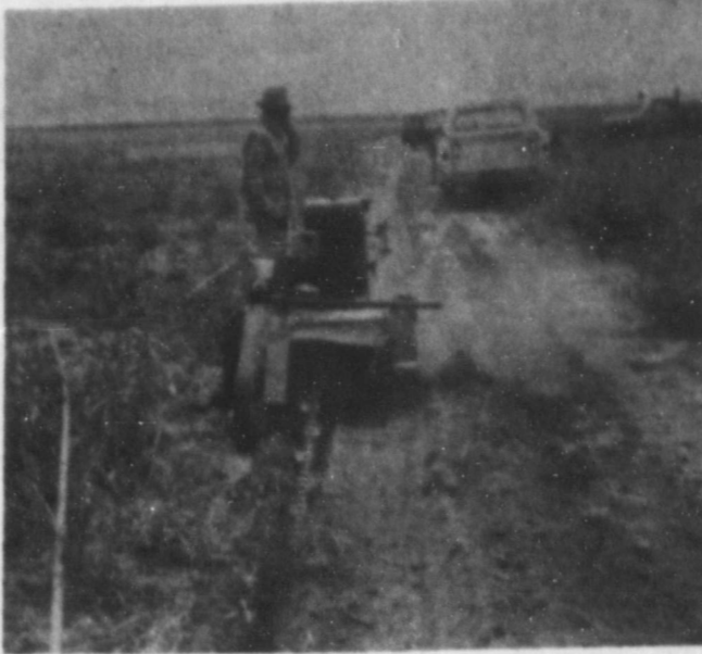
Picture above shows a livestock pipeline being put in on a local ranch. This pipeline will furnish water to an area where ponds could not be
