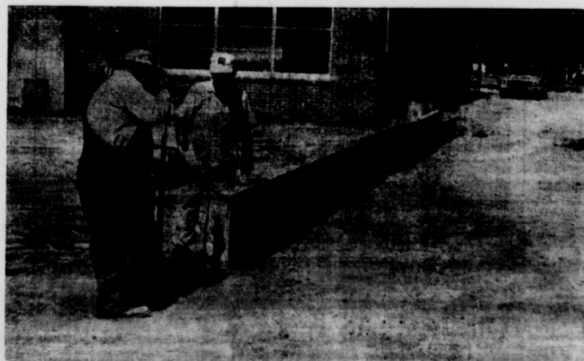
SIX NEW CLASSROOMS are being constructed at Burk Burnett Junior High School to take care of the expected increased enrollment this fall. Here the forms for the foundations are going into place. (Burk Star Photo)
