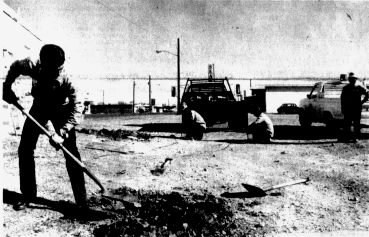
LEAKS, LEAKS AND MORE LEAKS — Darryl Boone, left, Alvin Dodson, Juan Becerra and foreman Santos Contreras of the city's water and sewer department were finishing up the last of the more than 50 water leaks they had repaired since the thaw of cold weather last weekend. They are shown here working off the 600 Block of the East Hwy. (SDN Staff Photo)
