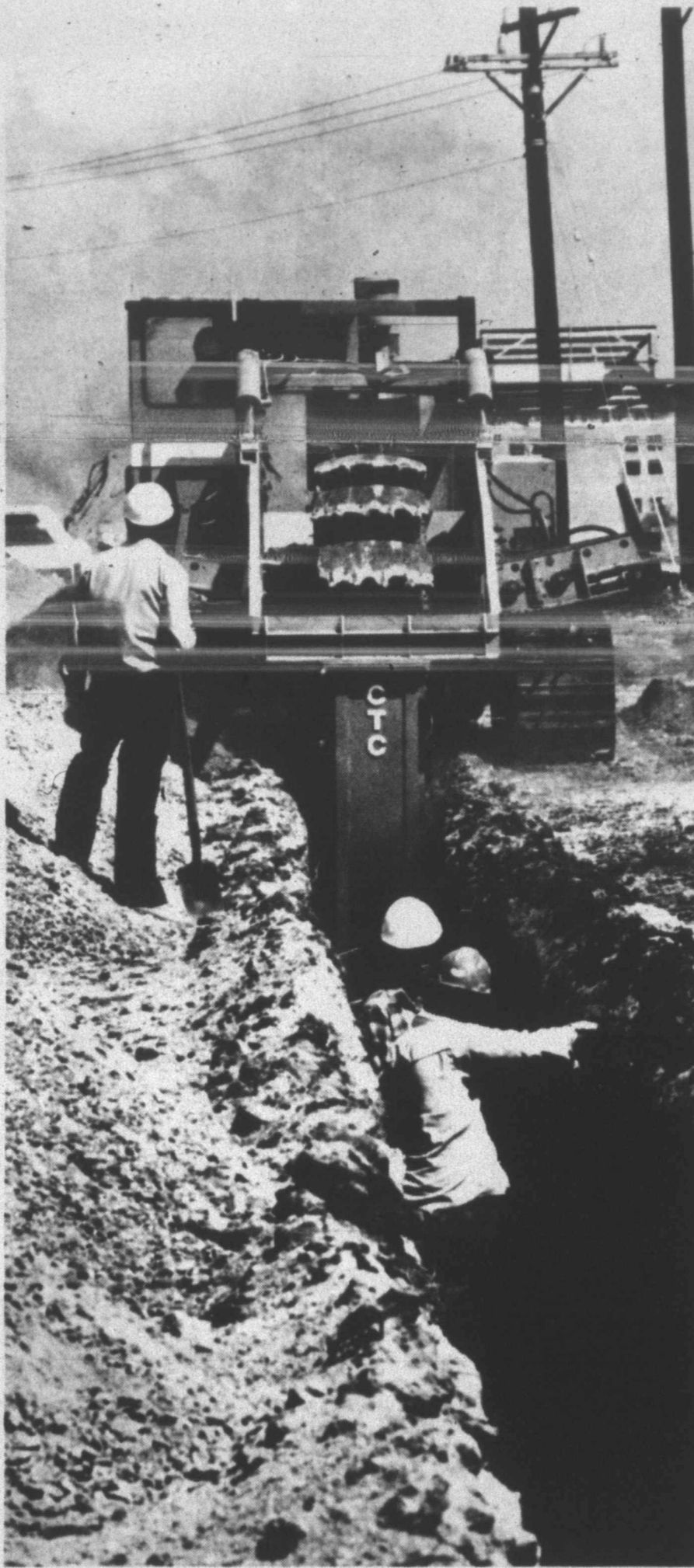
END OF THE LINE — The ditch digging crew laying a water line to the TDC Daniel Unit reached their objective on March 27 of this year. At this point, a similar line being laid for sewer connections was some 1½ miles still from the site. (SDN Staff Photo)
