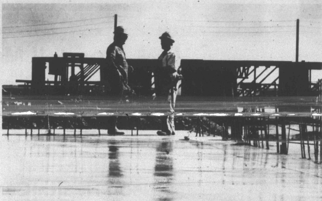
NEW CONCRETE — Workers had just completed this concrete slab at the prison site in early October of last year. At this point, some 200 workman were employed at the site. At its height, work activity was predicted at up to 250 individuals. (SDN Staff Photo)
