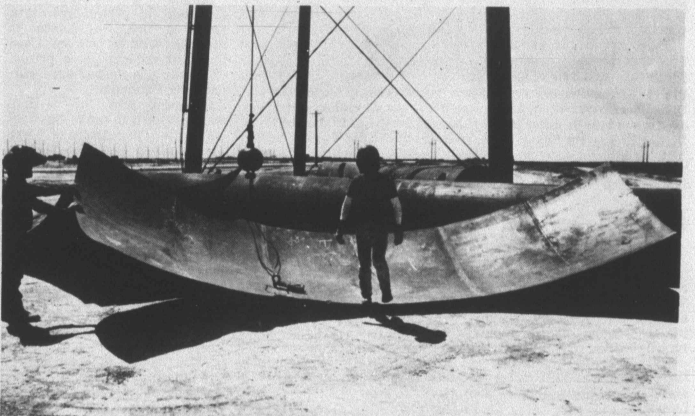
PUZZLE PIECES — Construction of the 150,000 gallon water tank at the prison site resembled putting together a giant puzzle in early April of this year. Worker Albert Peralez of Weslaco stands on one of the larger pieces. (SDN Staff Photo)
