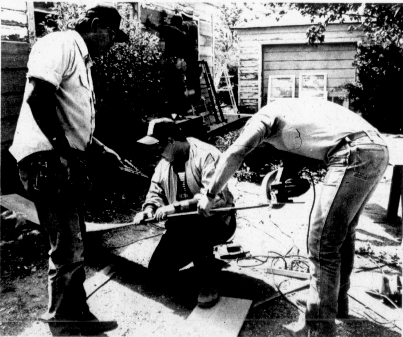
PANELING — Frank Ortegon, left, Rudy Garza and Wes Partain were cutting new paneling for a home as carpenters, painters and other skilled workmen worked to renovate homes throughout the city. (SDN Staff Photo)
