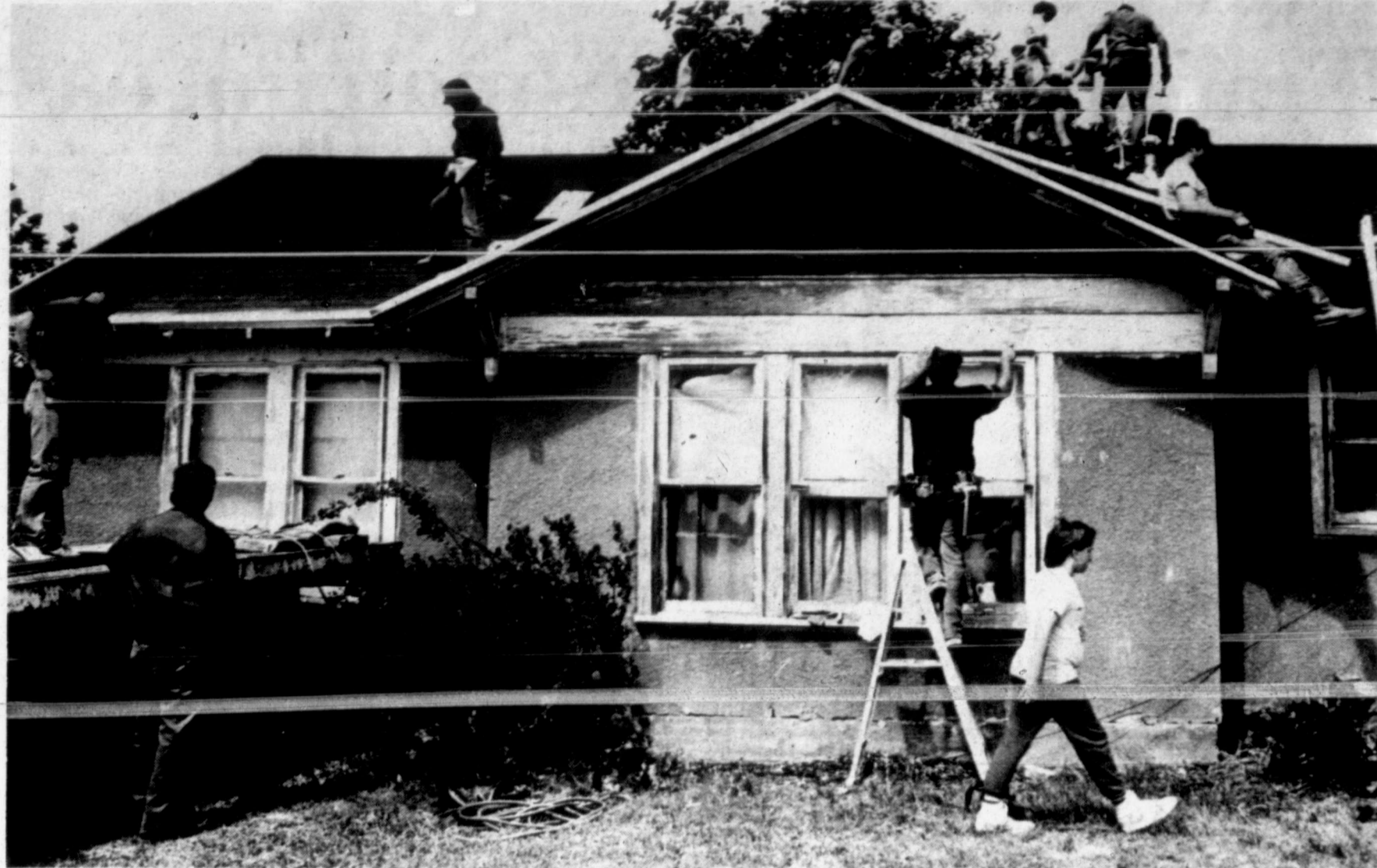
WHILE THE SUN SHINES — Volunteers for Snyder Neighbors Sharing were hurrying to make the most of the daylight hours during this one of the various one-day renovation projects undertaken Saturday by the group. (SDN Staff Photo)
