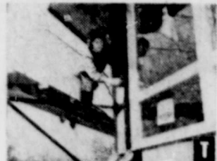
Finishing the construction work on their own homes gives single women like Margaret Bangerter much satisfaction. Here, she staples sheathing paper on her house before putting up the siding.
