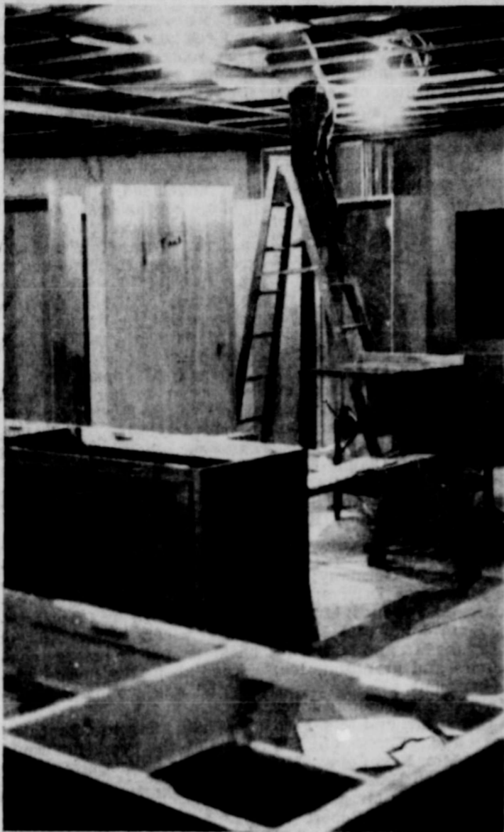
CEILING PREPARATION. The builders are winding up ceilings and accessories on school building.
