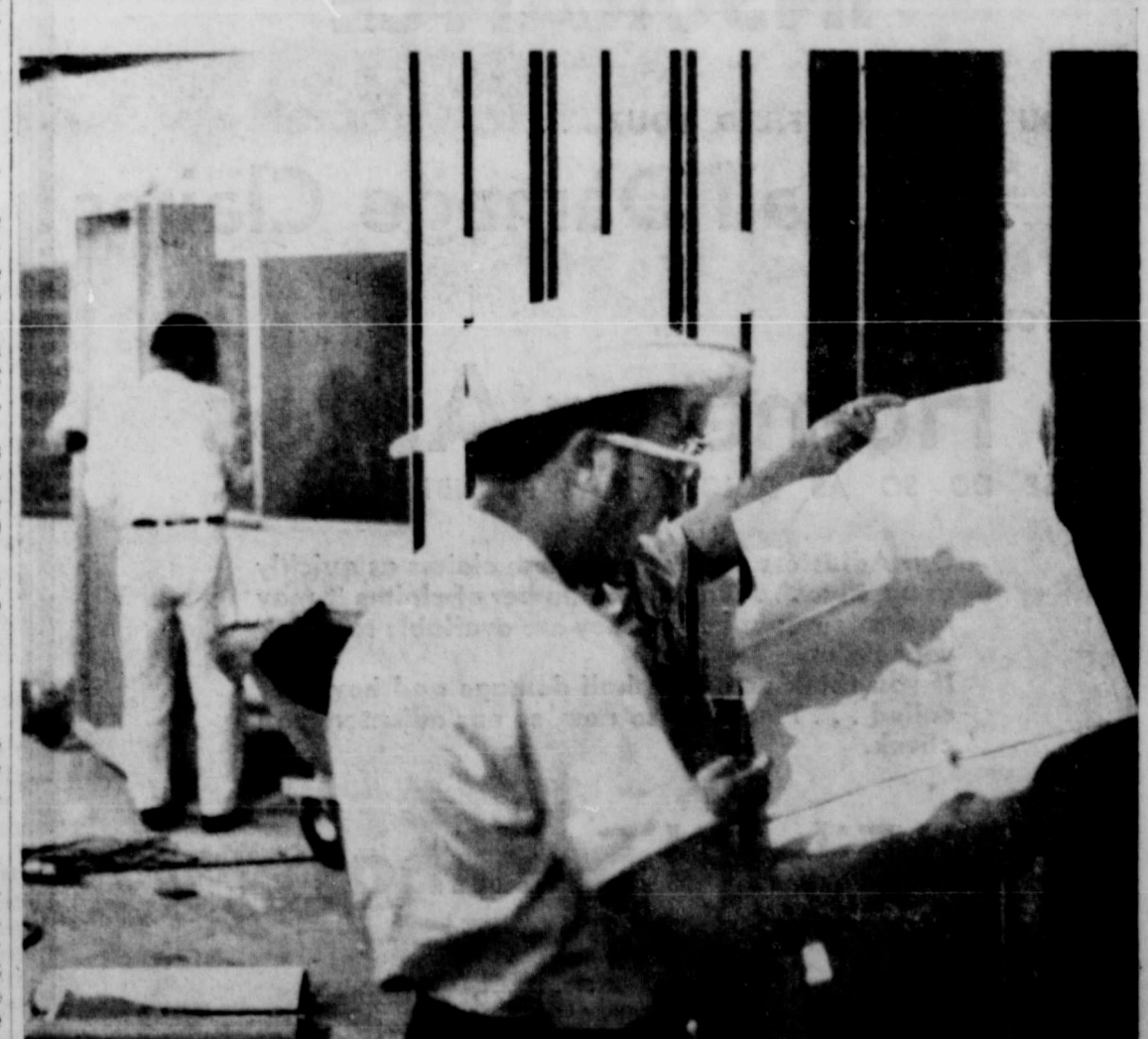
CHECKING THE BLUEPRINTS. Shown here are two of the builders checking the blueprints on the new school. The school is to be completed in time for classes this year. You may see more pictures of the new school on pages 2, 5 and 6.
