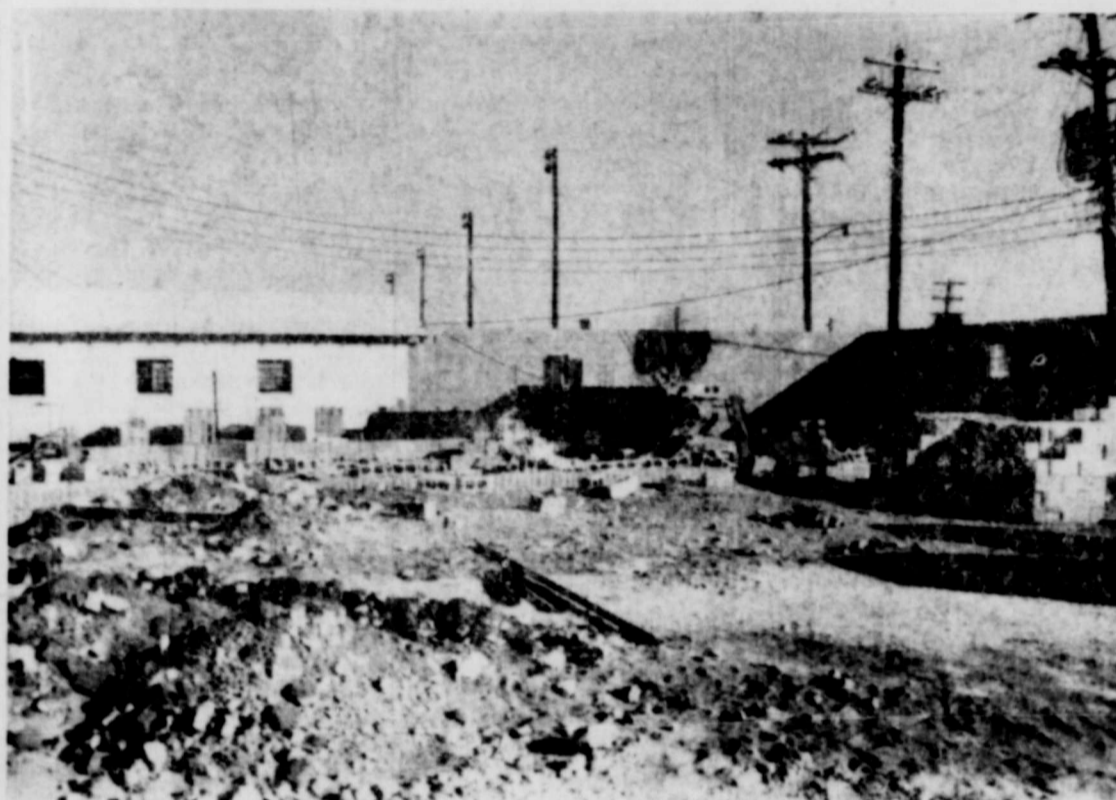
WIND BLEW IT DOWN—High winds last Thursday toppled the partially completed walls of the new field house being built at the high school. However, the damage has been repaired, and work is proceeding rapidly towards completion.
