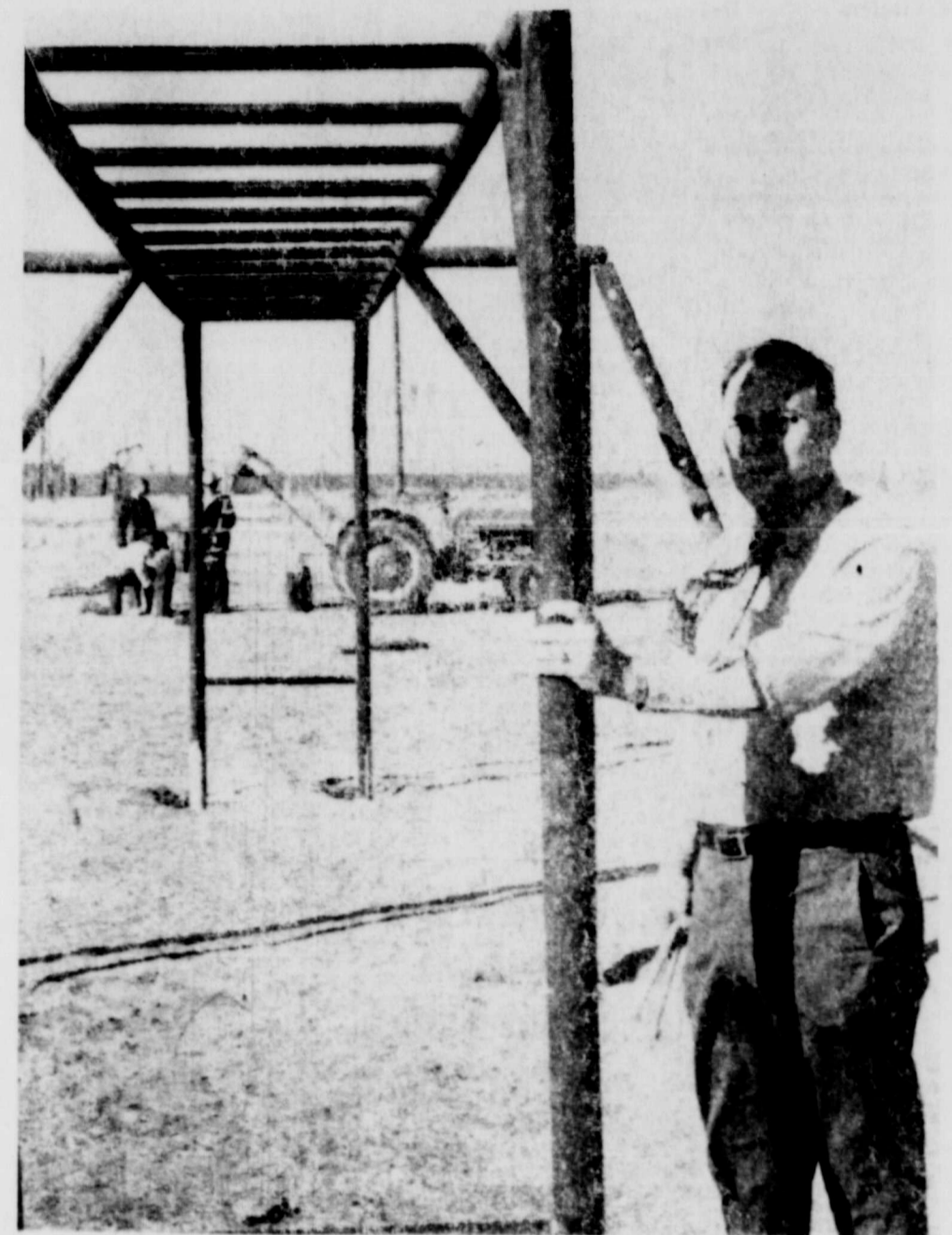
LENDING A HAND—Football Coach and Athletic Director Bill Young lends a hand during recent construction of the new track and obstacle course at the high school.
