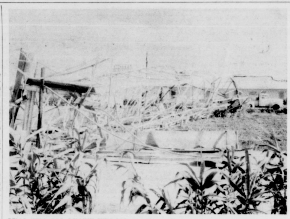
BELLS TOLL FOR BELVUE SIGN —The weather bells sounded finish to the big sign symbolic of oil production in the area and located on Motel Belvue Restaurant grounds late Tuesday night. The derrick type structure with the revolving beacon flasher at the top hit the soil with a dull, muffled thud. The windstorm had deprived highway travelers hunting for overnight accommodations and airplane pilots flying overhead of a monumental direction signaler with just one strong thrust of power. The sign will go back up soon. That's a promise from Mr. and Mrs. Roy Kelly, owners of Motel Belvue.
