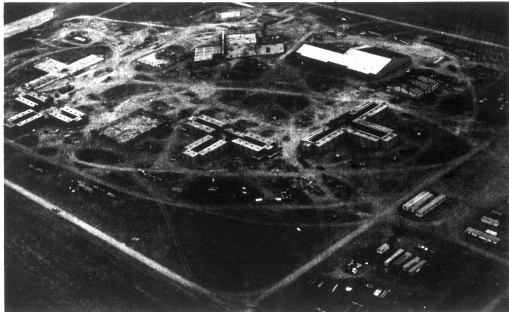
BIRD'S-EYE VIEW — County sheriff's deputies Andy Anderson and Darren Jackson, flying in Anderson's airplane, caught this aerial view of the Texas Department of Corrections construction site east of Snyder late last week. The big building with the broad roof at the
