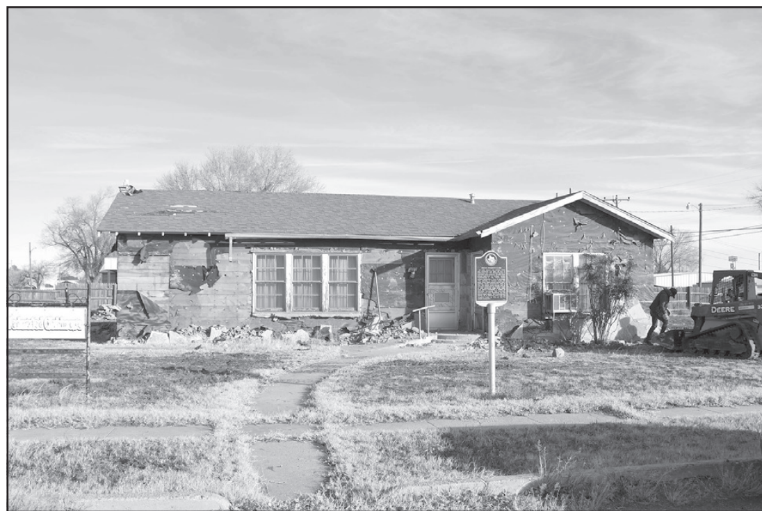
Work is underway at the Women's Federated Clubhouse just north of the Methodist Church. The rock exterior was removed and will be repurposed.
