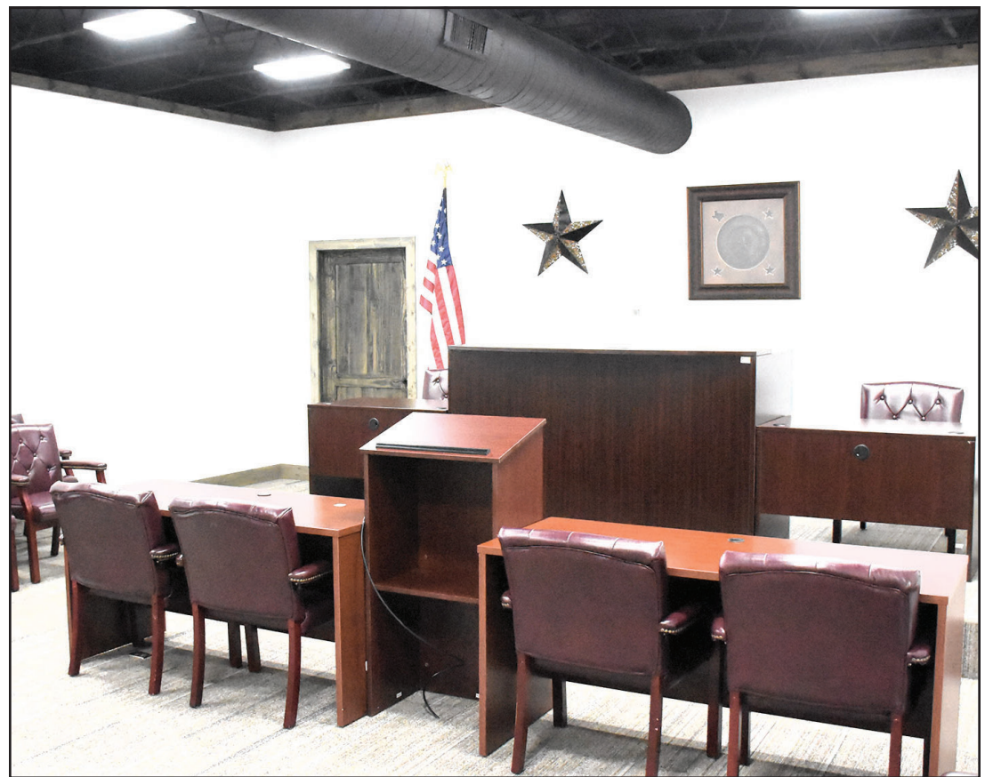
Construction is nearing completion on a new courtroom at City Hall located just south of the City Council Chambers and is accessed by using the south door facing Main Street. The new facility will be home to the Friona Municipal Court Judge Deborah Campbell and Justice of the Peace, Precinct 1 Rhonda Wilkins.
