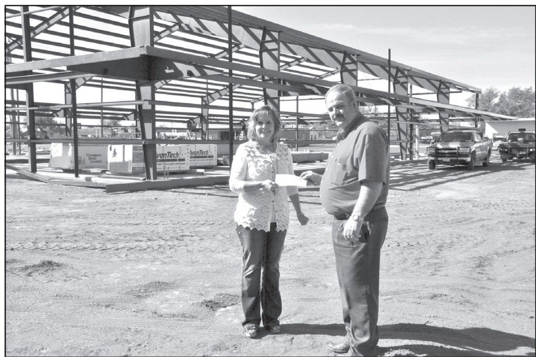
Parmer County Farm Bureau manager Mitchell Smiley presents a $500 donation toward the Bovina community center building to Bovina city manger Jana Pitcock. The steel is up on the building, located next door to the Bovina city hall. The center will include a gym, kitchen, and space for meetings. Ron Carr photo. (Friona Star, Thursday, April 12, 2012)
