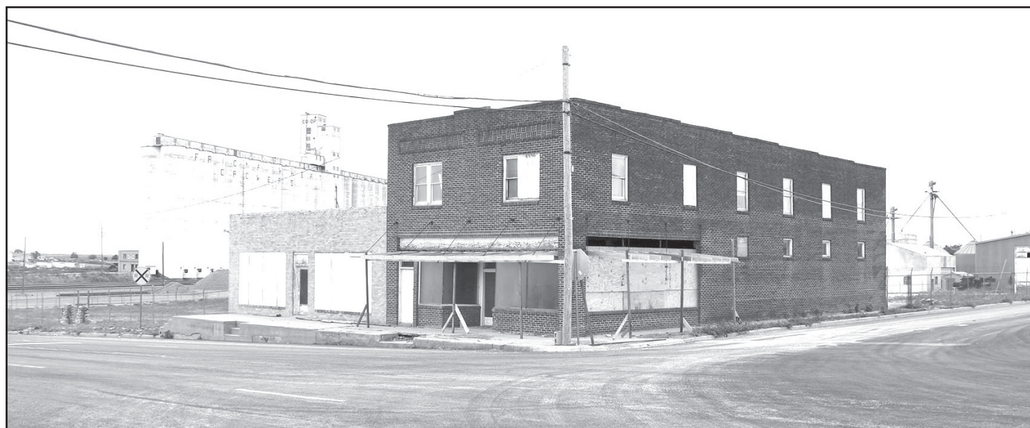
Renovation has begun on the Mauer building at 5th and Main. The two-story building was built in 1928 and was home to Mauer Machinery until 1973. It is the future home of The Farmwife Kitchen restaurant currently located on the west end of 5th street. Plans are to open sometime near the first of next year.
