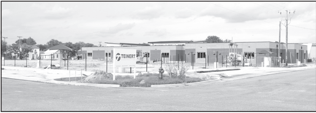
The new Primary School is under construction. The rain has led to a slow installation of equipment and the new playground but things are back on track.
