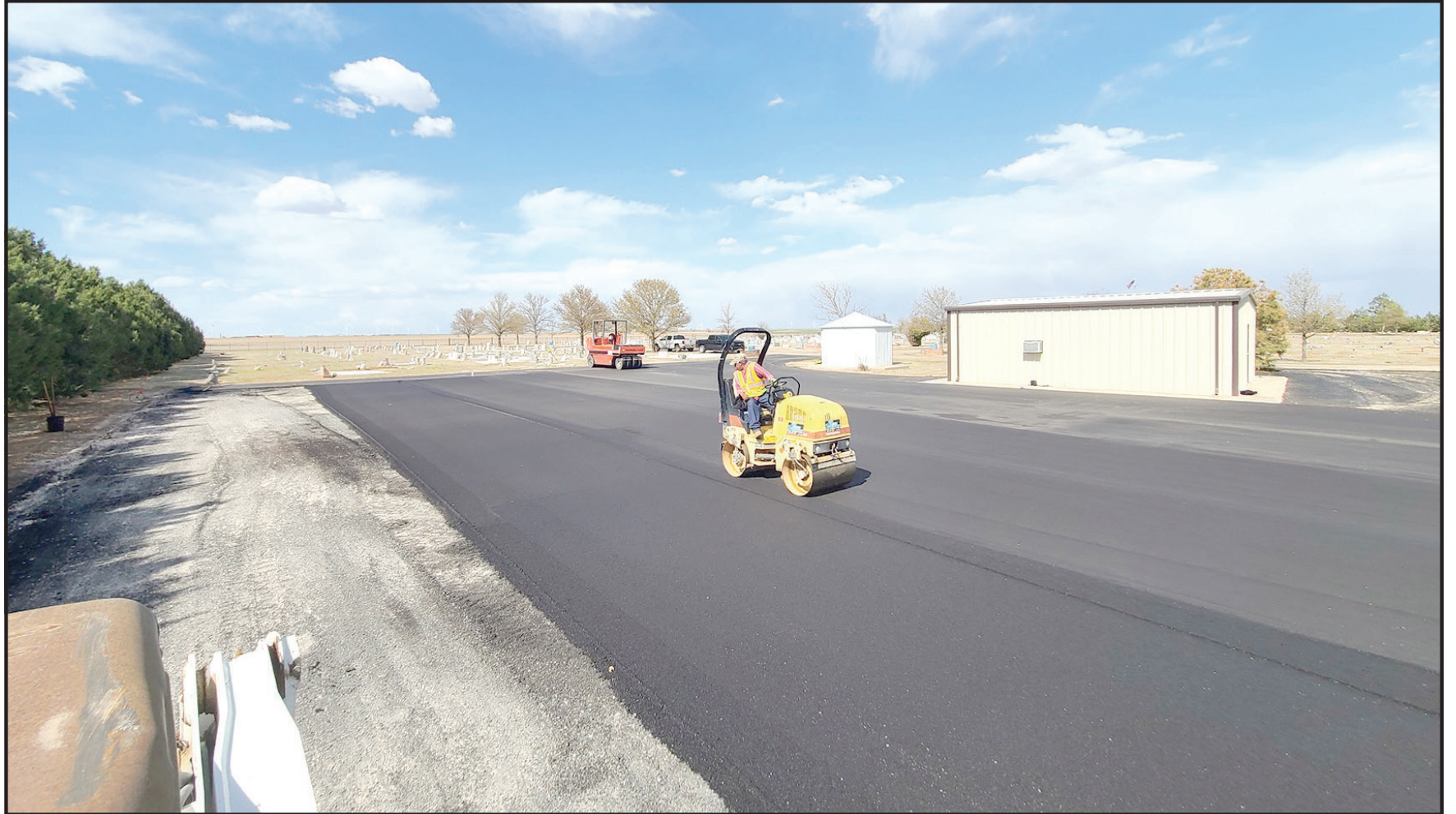
Bermea Construction is nearing completion on the new parking lot around the Chapel at the Friona Cemetery. The existing roads at the Cemetery will also be resurfaced as part of the project. Photo courtesy of Bermea Construction
