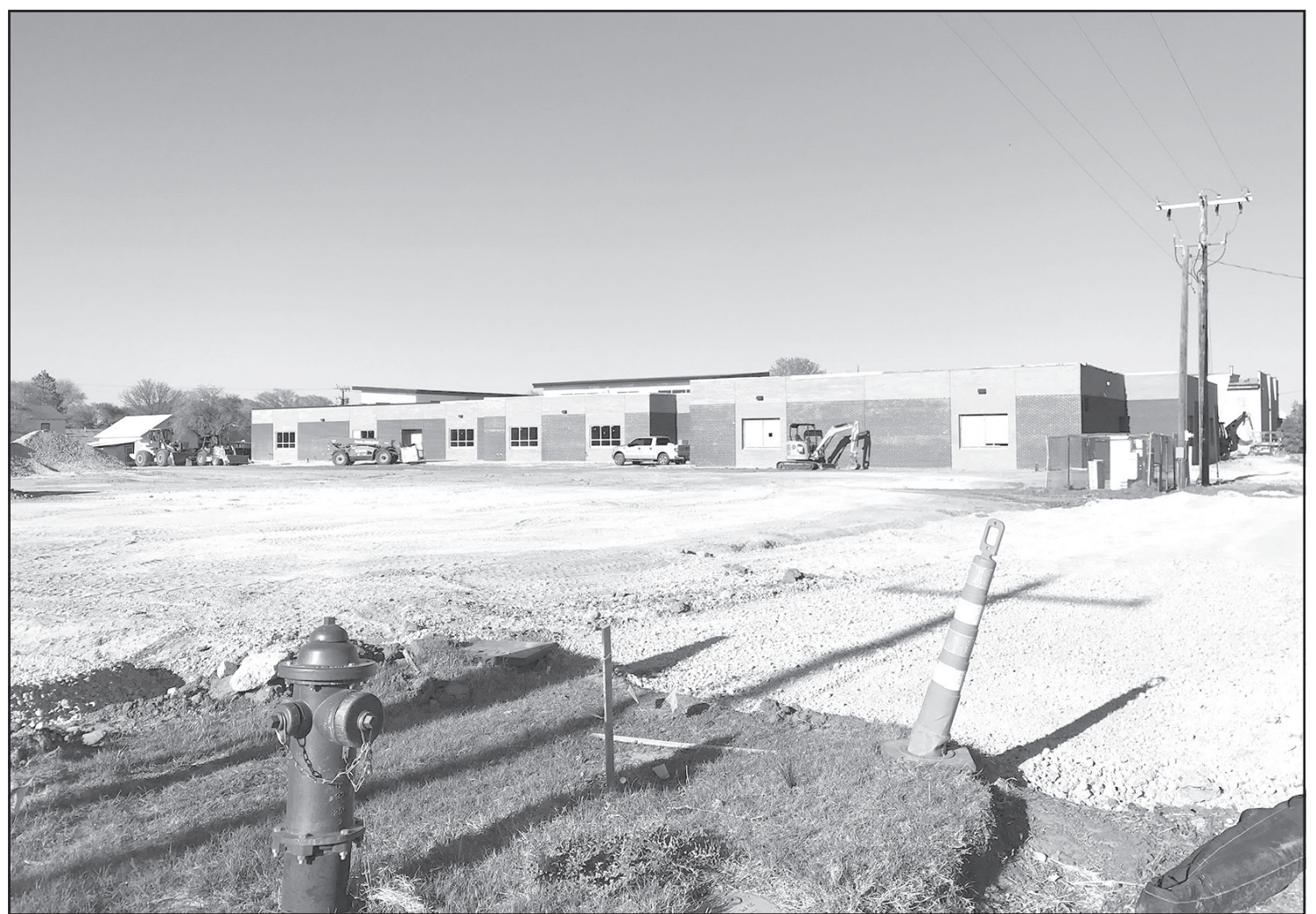
Teinert Construction will finish work on the new Primary School building in the next 3-4 weeks. This photo of the west side of the new facility also shows the empty lot where work on parking, playground, and general landscaping will soon begin.
