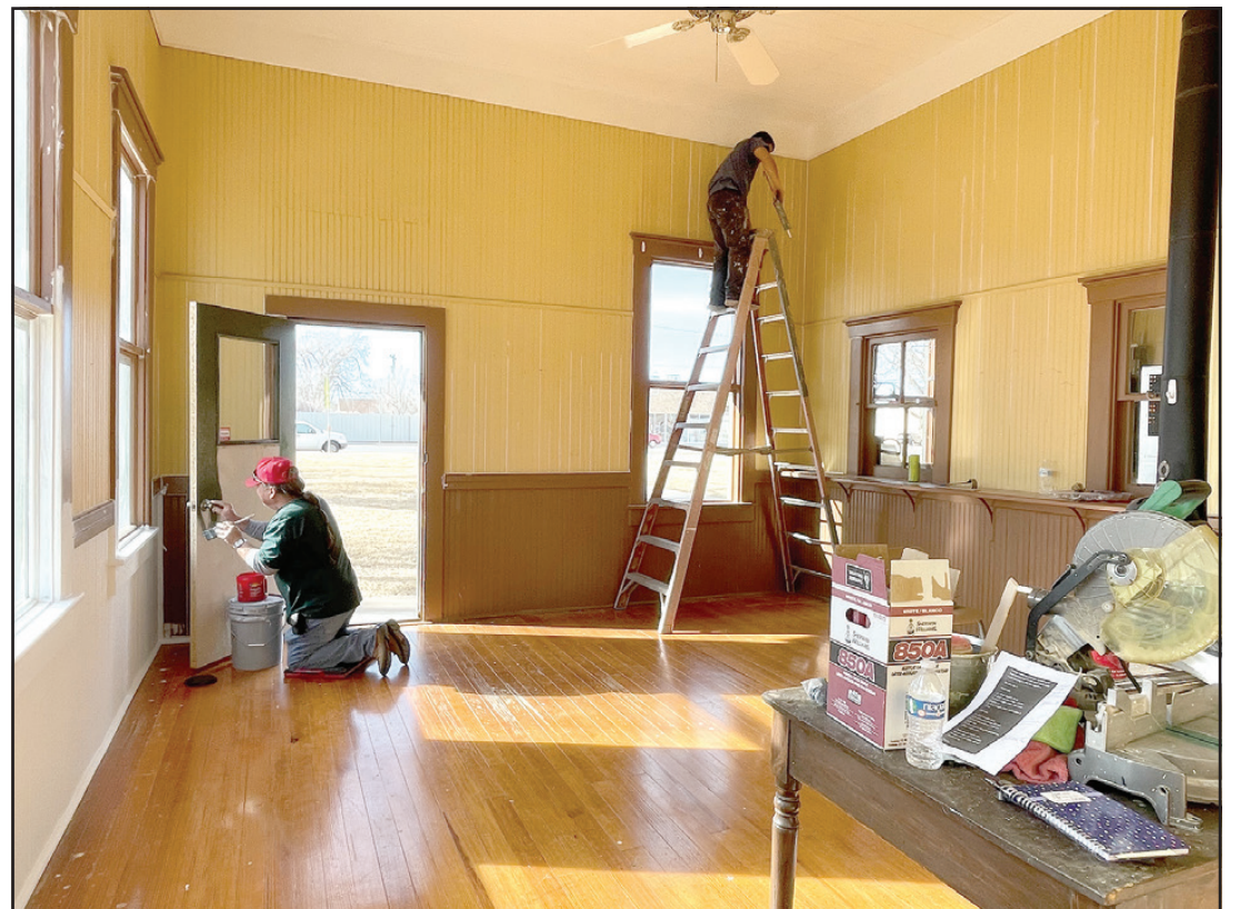
Johnny Alvarez, and crew, have been refurbishing the Depot the past few weeks. Birds had found their way in but could not get out and therefore caused quite a bit a damage. The outside of the Depot will also get a facelift as soon as the inside repairs are finished and warmer weather arrives. Courtesy photo. If you would like to make a donation to help with repairs you can contact Jeri Lynn White.
