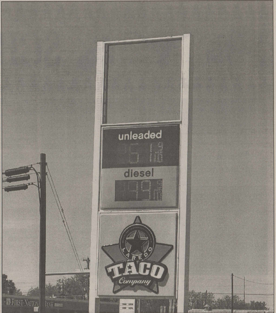
Something's Missing! A storm rolled through Bronte Tuesday evening, April 24, 2018, that included some high wind gusts. The winds with this storm resulted in the loss of the top portion of the Stripes sign in Bronte.
