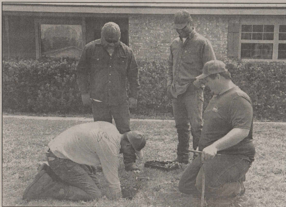
New Meters! Robert Lee city workers and others worked in yards and alleys replacing the old water meters with new digital meters. The new program is the result of a 70/30 grant received by the City of Robert Lee for this purpose.
