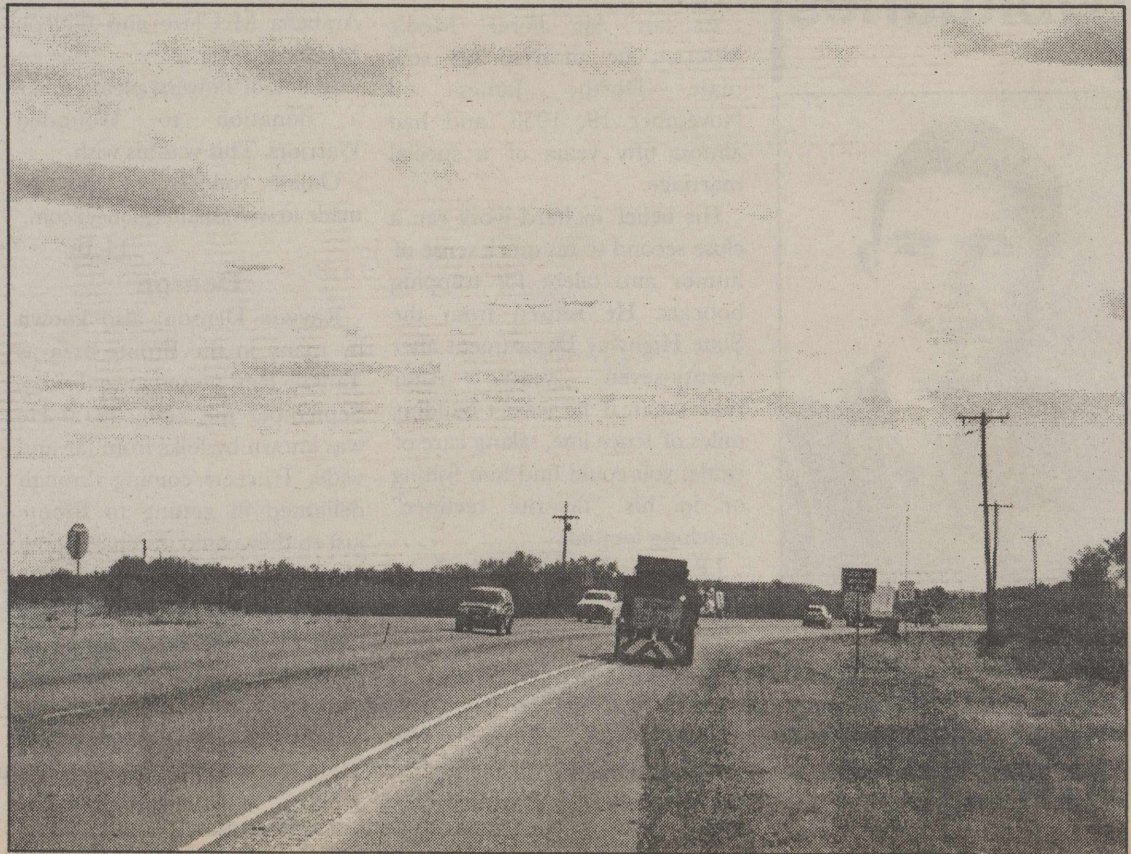
Highway Safety! TxDOT crews were out in force Monday, October 5, 2015, adding safety features in the four miles of US Highway 277 just north of Bronte. They first brought in a radar trailer a couple of weeks ago and this week, they cut in rumble strips. The strips run just outside of the white lines and down the center of the highway.
