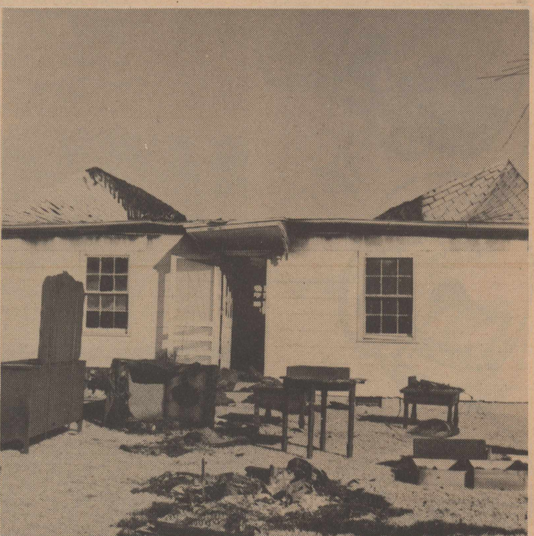
This was the scene last Thursday morning after the Jimmy Ivy family had suffered a disaster by fire. They were rejoicing that neither they nor their four sons were inside the house. "We drove up to the house a few minutes after 7, and smoke was pouring from the eaves. We had a fire extinguisher and had hooked up a hose, opened the back door and flames immediately filled the doorway," said Mr. Ivy. The Seminole Volunteer Fire Department arrived in record time but very little could be done to save clothing, furniture or house. Evidently the fire started around the cook stove as the floor was burned out there. The roof of the house fell in, as seen in the picture. Mr. Ivy is employed by the Great Plains Water District, Inc. and lives 13 miles down the Frankel City Highway and 2 miles south.
