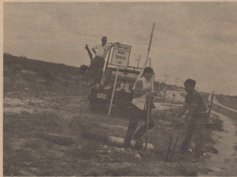
An accident that claims lives many times causes other property damages. Colonel Rambo, Jr., Danny Butts and Dwain King can be seen here as they replace highway markers and two signs on FM Road 1757. In the background can be seen the telephone company's truck where poles had to be replaced, also a fencing crew rebuilt 75 feet of fencing that had been torn down.
