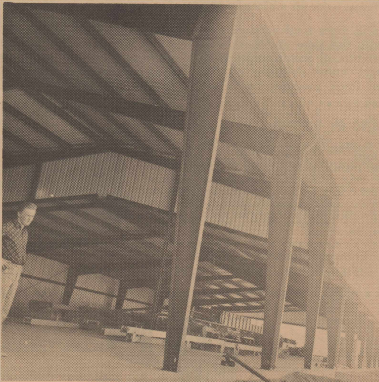
Jouni Sarkkila is standing in the new packing shed at the Wolfe Peach Orchard. The main building measured approximately 60 ft. x 220 ft.
