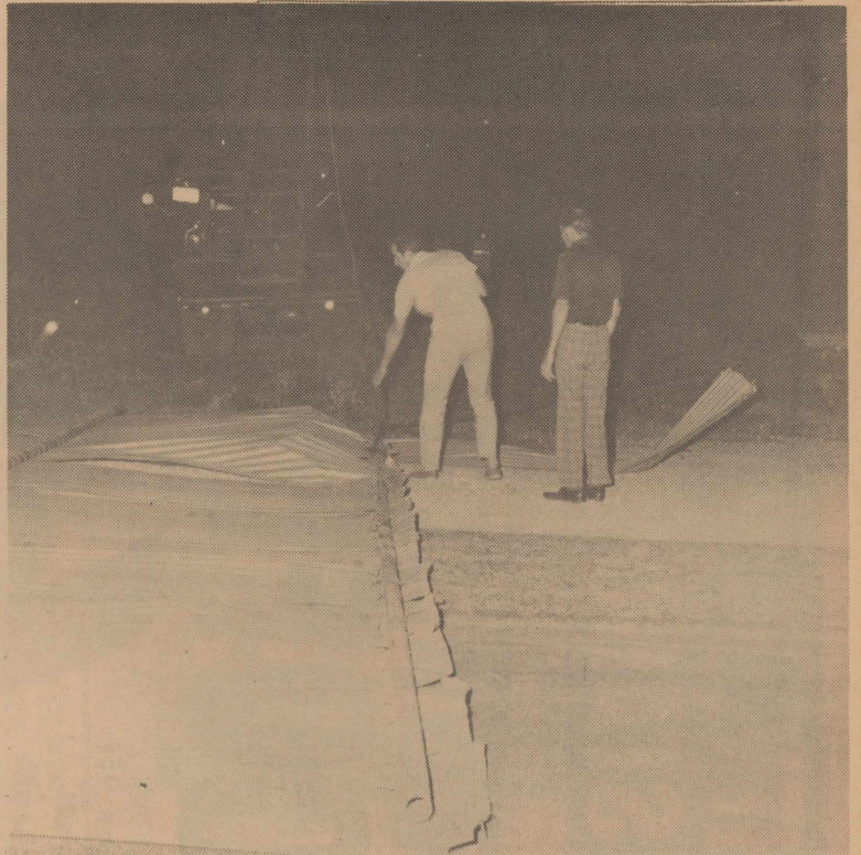
JERRY LEGARD AND C.D. WICKSON JR. ACT AS SWAMPERS LAST WEDNESDAY NIGHT AFTER THE STORM IN TRYING TO REMOVE AN 80' SECTION OF AN AIRPLANE HANGER OFF THE HIGHWAY. DALE JOHNSON OWNER IS OPERATING THE TRUCK.
