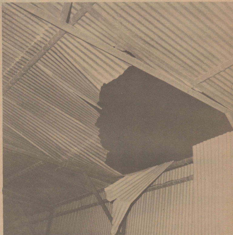
A GAPING HOLE IN A HANGER BUILDING AT THE AIRPORT AFTER LAST WEDNESDAY NIGHTS STORM.
