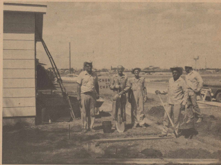
The 7th Street Church of Christ is adding 840 square feet onto their present building. Shown working on the buildings left to right are Junior Hilton, Jim Stakely, Rupert Caffey, Augustin Rascon and Jesse Alvarez.
