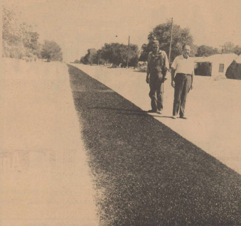
Mr. C. A. Tubbs, engineer, views the last coating going down on 11th Street along with Mr. A. L. Haller.
