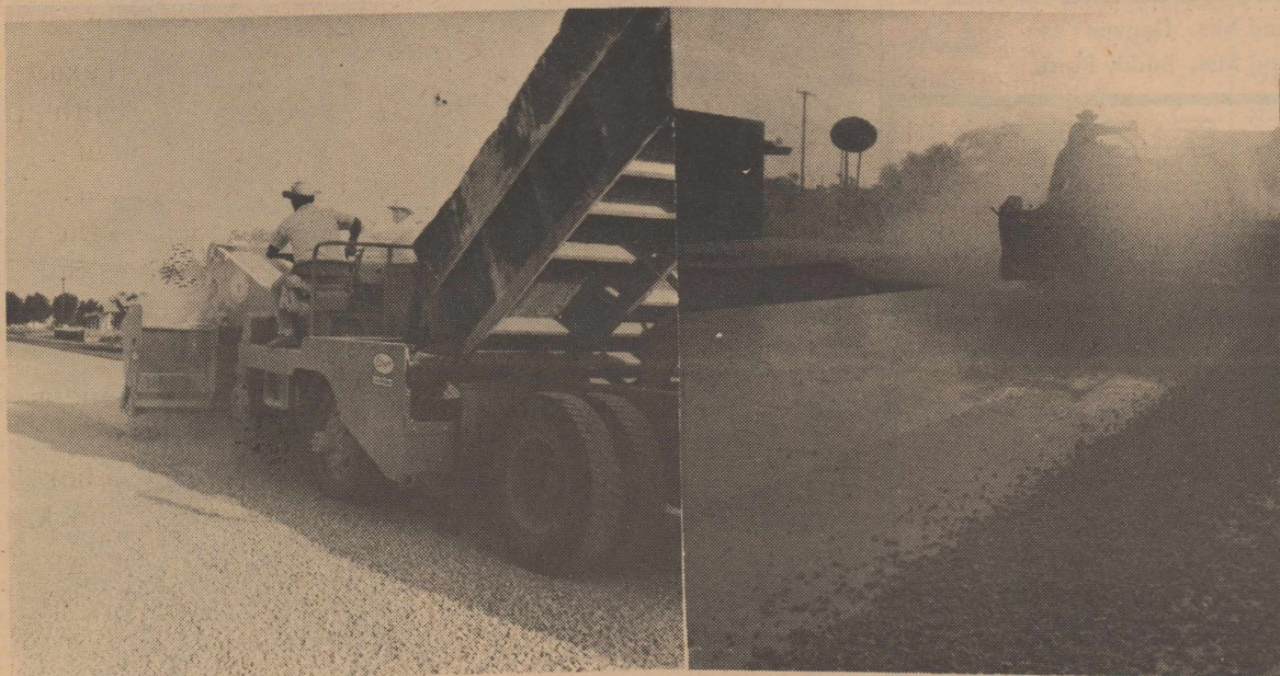
FINALLY, FINALLY - early and late, the paving crew is finishing up some of the streets in Seminole. This scene is on N. W. Ave. B. with Production Credit in the background.
