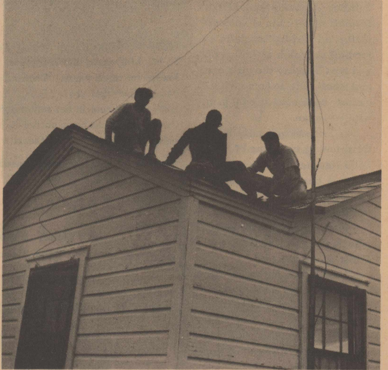
Don Moore, Howard Farmer and Jimmy King are working late hours in the 500 block of 10th Street, repairing a rent house.
