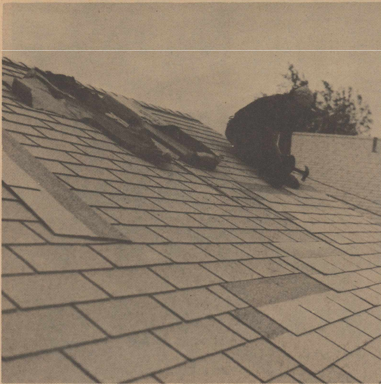
A DO-IT-YOURSELF PROJECT --- Dupree Woodruff is hard at work at 806 SW Ave. D. recovering the roof after the hail damage.
