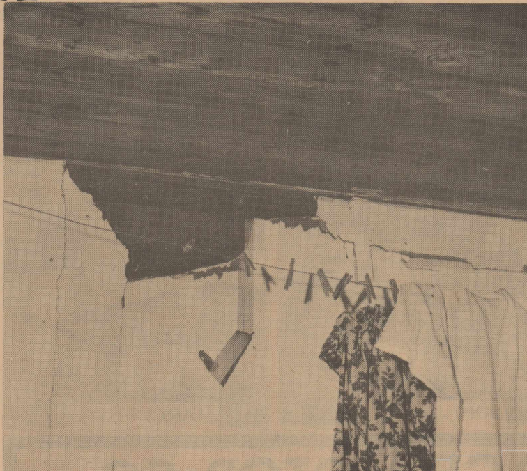
Daylight can be seen between the ceiling and the wall after an explosion which caused the sheetrock to burst at the L. E. May residence, Denver City Highway.
