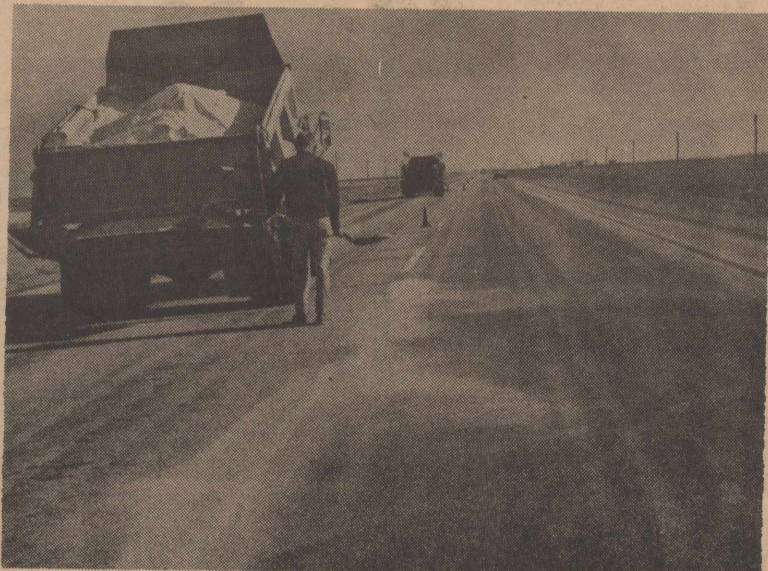
Highway 285 around McAdoo curve is being patched. The cracks are being filled with asphalt then rock dust put over it.
