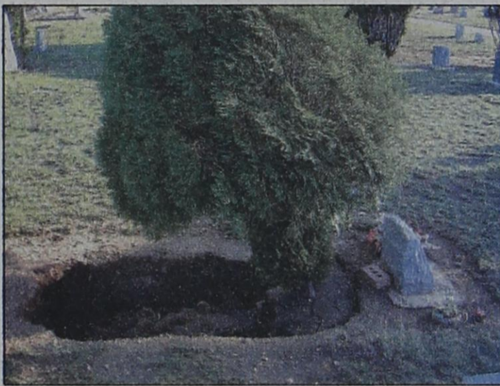
Sunken graves — Severe rain caused approximately 55 graves in the Bailey County Cemetery to cave in. Members of the Cemetery Association spent their weekend restoring graves such as this one.
