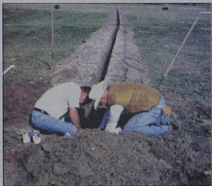
Diggin' a ditch — David Brunson and Don Sharp (pictured respectively) along with other Rotary members dug a ditch for a drip irrigation system at the City Park Saturday morning. The Rotary Club plans to plant shade trees at a later date as a community service project. Other members helping that weekend were George Nieman, Lary and Wanda Hooten, and Mike and Chris Cleavinger.
