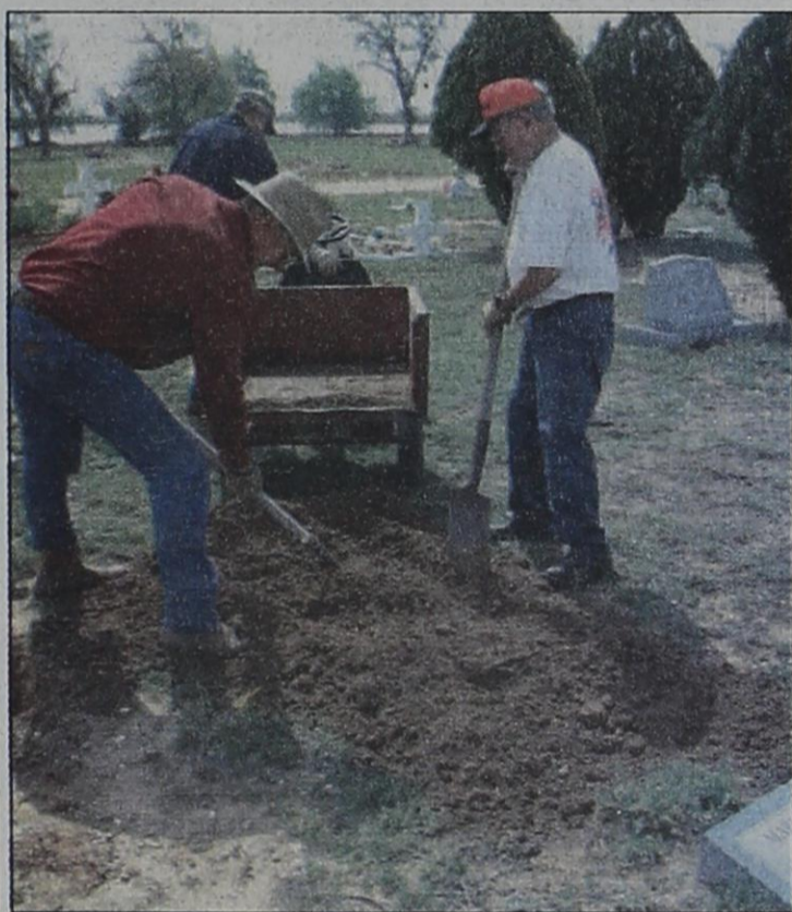
Graves restored — Marshal Head (left), Paul Poyner (right) and David Weir (middle) were among the Cemetery Association Board members helping restore grave sites this weekend after rains hit the area, destructing several sites at the old cemetery.
