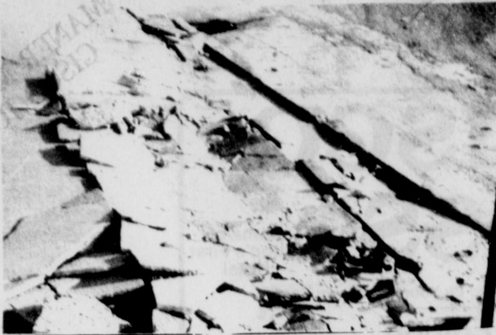
DAMAGED SIDEWALK-- The sidewalk in front of Dixon's Auto Supply was crushed Tuesday night when a huge truck tried to turn onto East 6th Street from Conrad Hilton Avenue. The truck was attempting a wide turn when the wheels ran over the sidewalk. The city will get estimates on the damage and the trucking company's insurance will pay for repairs. (Staff Photo)
