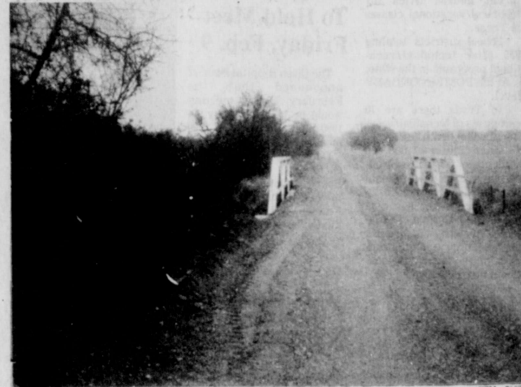
The new bridge is in -- the sides are painted. Twenty-one yards of concrete were poured on this one. It ought to last a long time.
