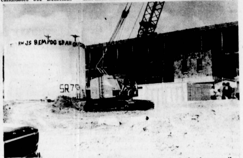
ONE OF FOUR valves inside the dam were being looked at by council member Ivan Webb and Mayor Eris Ritchie when the above photograph was taken Saturday morning. City engineering firm's representative, Ken Martin, told the group that the valves will be replaced during the construction. (staff photo)
