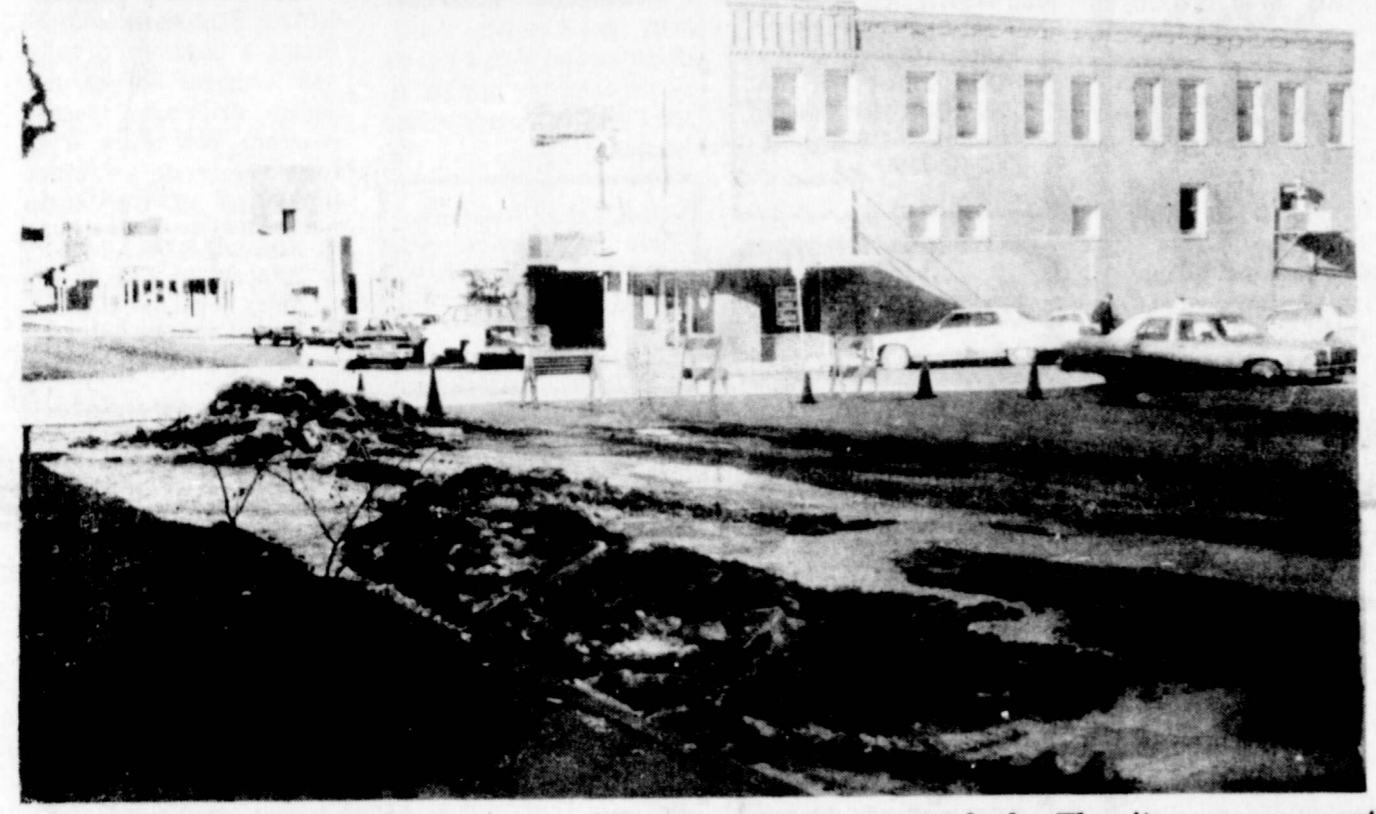
WATER REPAIR CREWS of the City of Cisco were working in 700 block of Conrad Hilton Avenue last Friday afternoon on one of numerous water leaks. The city crews are continuing their work of repairing water leaks during warmer weather. (Staff Photo)
