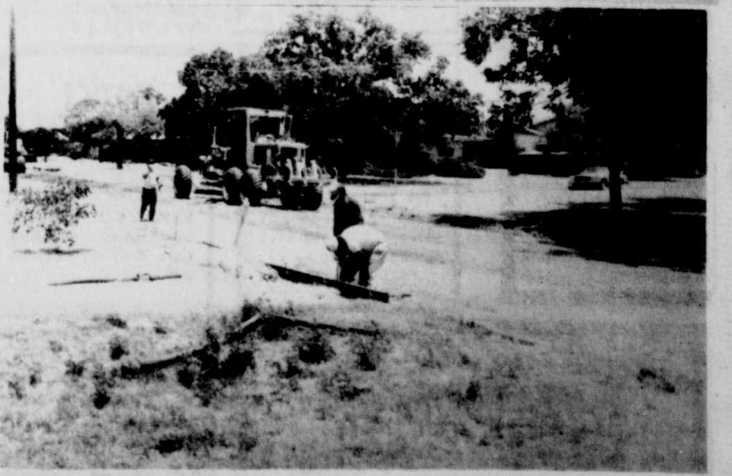
Crews of the Zack Burkett Company of Graham are working on the City of Cisco's paving project on Front Street from West 8th to 2nd Street. The brick pavement has been removed and will be replaced with gravel. Curb and gutter will also be replaced in the area of the brick pavement. (Staff Photos)
