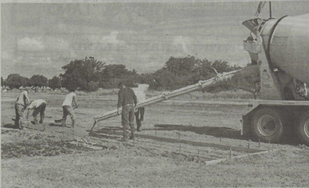
Pouring Concrete - The concrete is being poured for the new helipad at the Cross Plains VFD Fire Station. Made possible by a generous donation from Comanche County Electric Coop, the helipad will make it easier and safer for the AirEvac helicopter to land and take off in Cross Plains.
