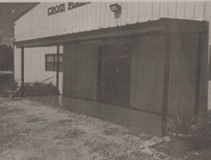
The Front of the Firehouse has a new look with a concrete slab at the entrance
