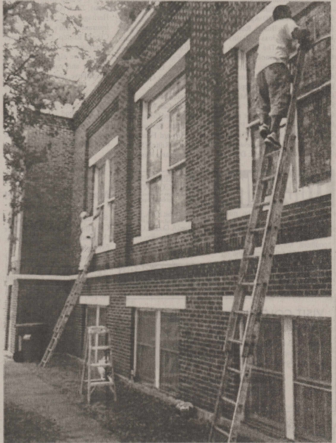
ABOVE IS A PICTURE OF WORK BEING DONE ON THE OUTSIDE WINDOWS!
