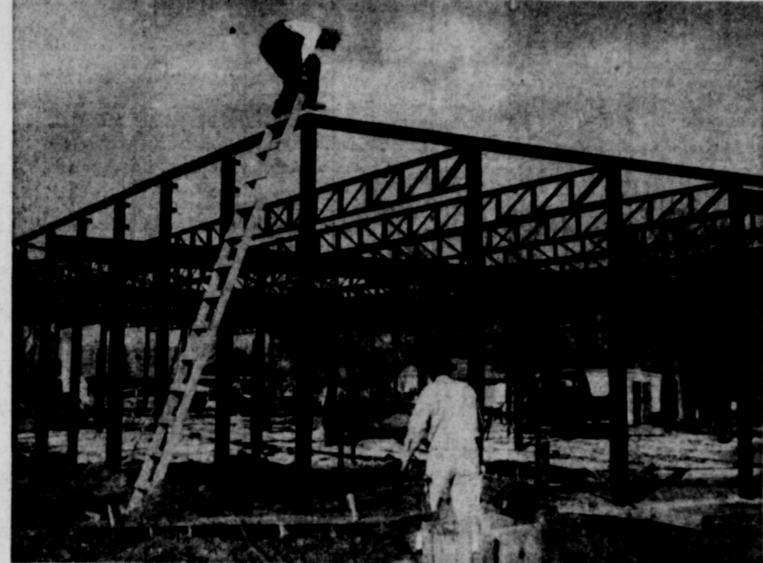
CONSTRUCTION gets well under way on the new vocational agriculture building at the High School. The building is to be ready for occupancy prior to the beginning of the next school term. (Advocate Photo)
