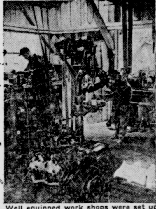
Well equipped work shops were set up for repair work as well as centers for extensive construction at the airports.
